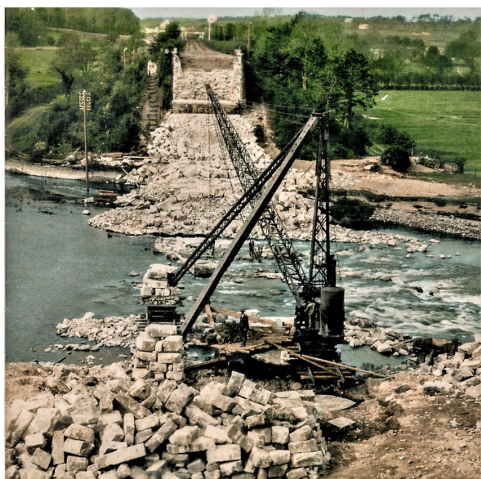
Figure 5 The destruction of the Mallow Viaduct which was not repaired until Oct 1923
